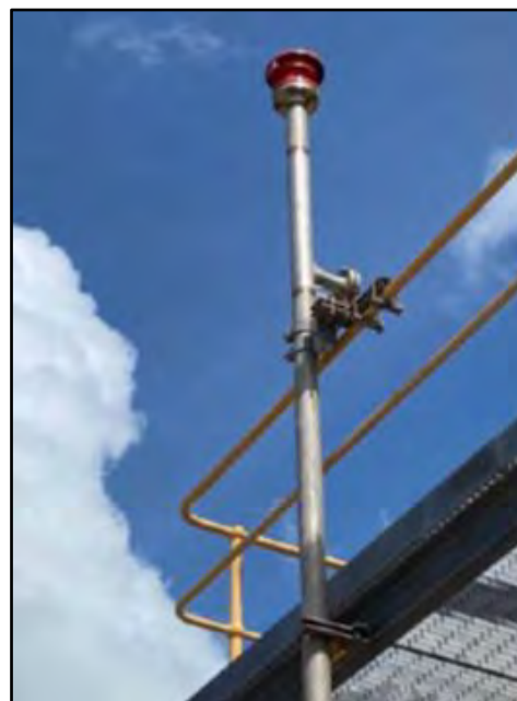
Figure 2: Scrubber Vent Stack
