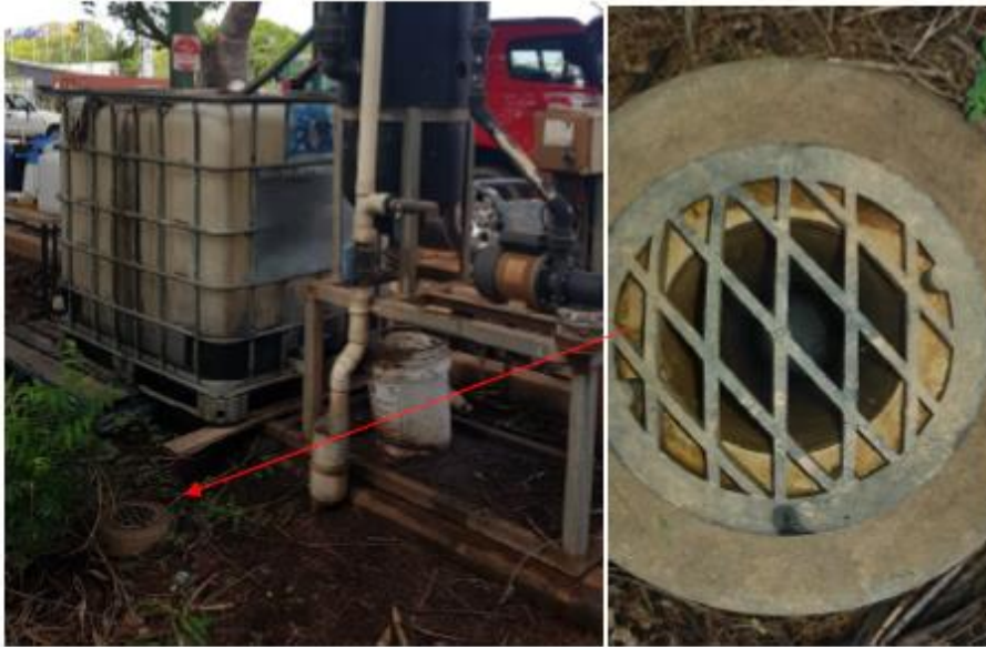
Figure 4-3 Sample Point for the Vertical Gravity Separator (grate to be removed during sampling and then replaced)
