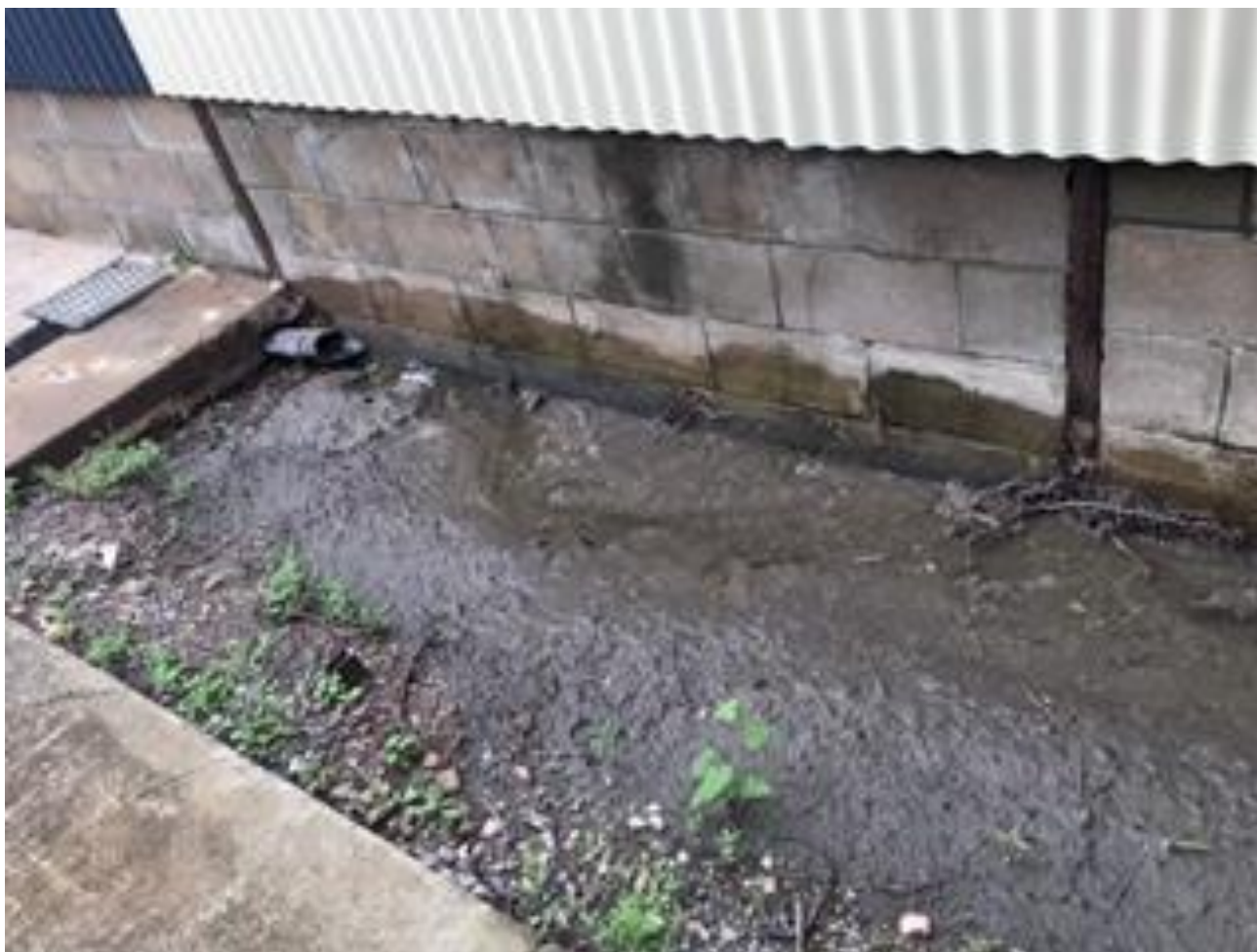
Appendix B – Photographs – Spill site, ORG on northern side of residence.
