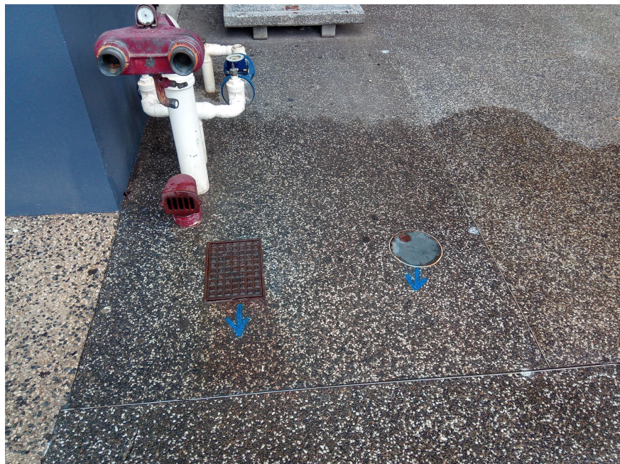
Property micro-flap vent and inspection shaft, from which discharge occurred.
