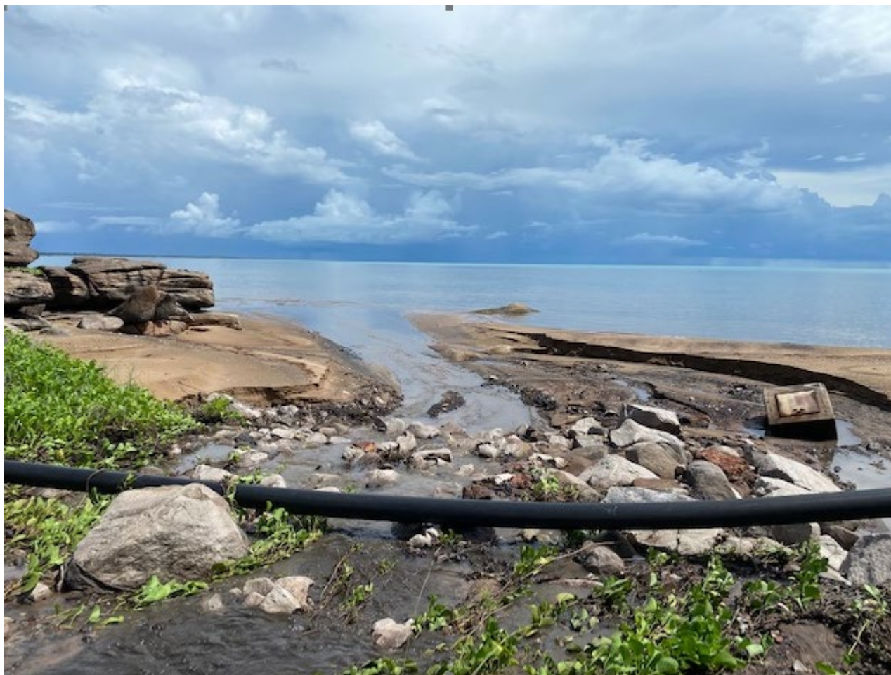
Figure 3: Photo taken after the incident looking out at the Stormwater release point. Photo taken at 2:25pm.
