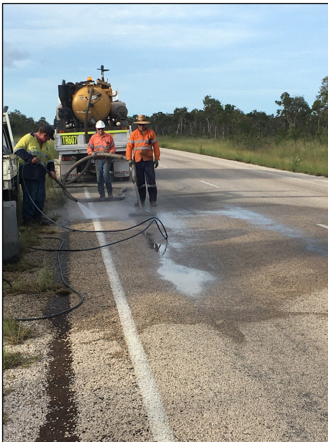
Figure 3: Spill clean-up efforts via pressure cleaner and industrial road sweeper at site 2.
