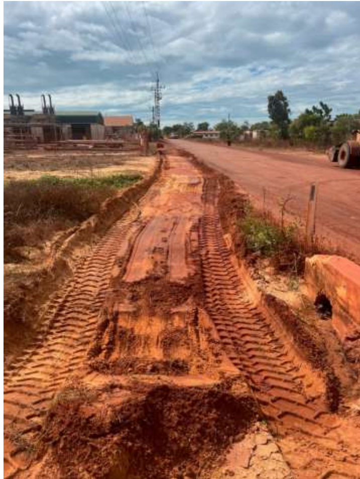
Pic 3: During clean-up along roadside
