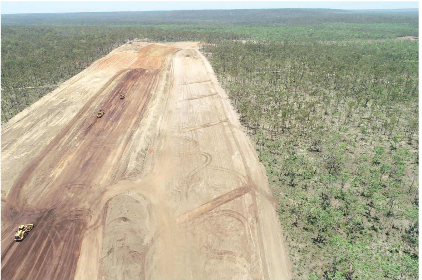
Figure 8: Improved ESC: Increased frequency of diversion bunds along the haul road.
