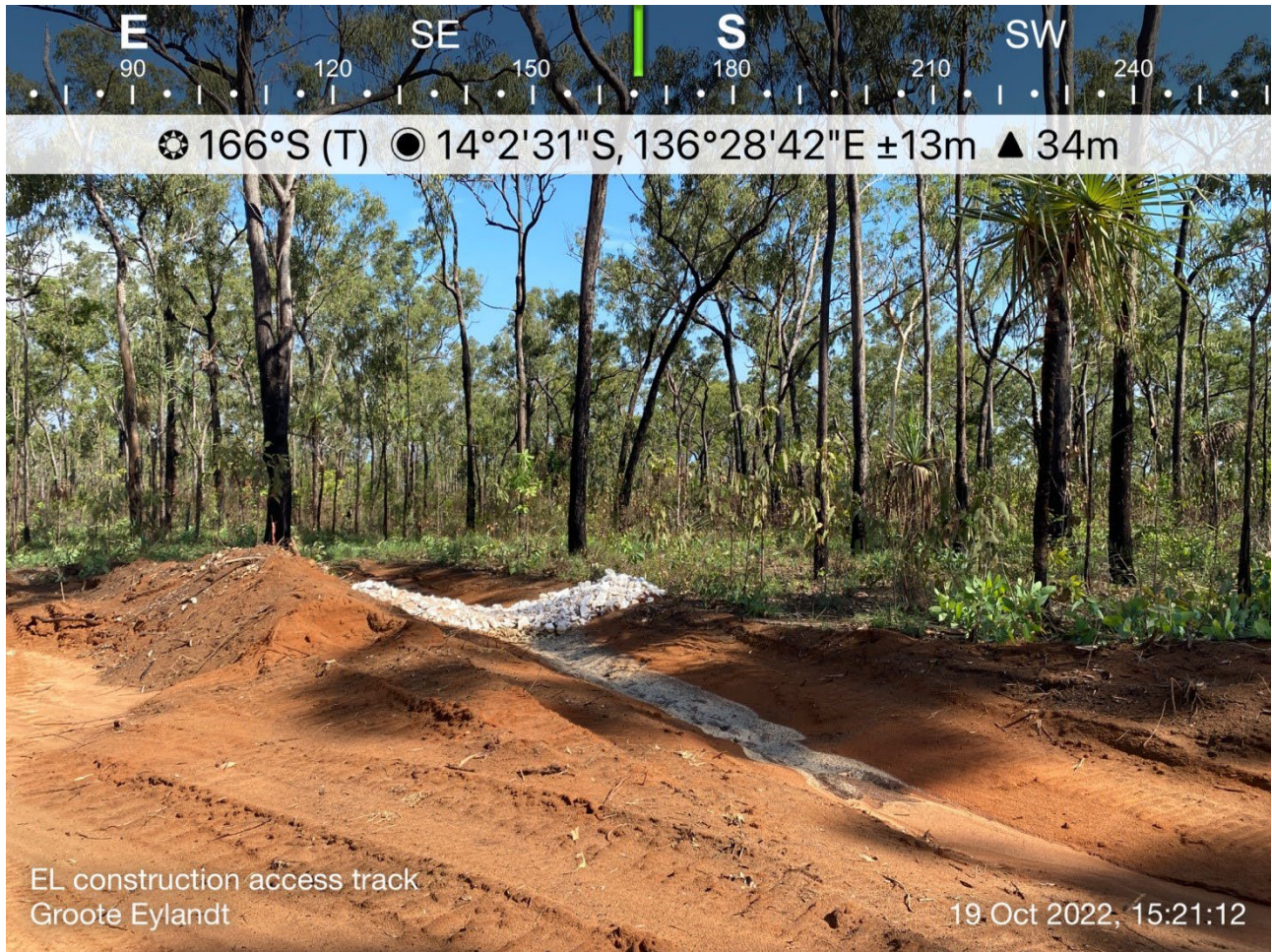
Figure 6: Temporary ESC at the time of the event: Stabilised outlets from the construction access track.
