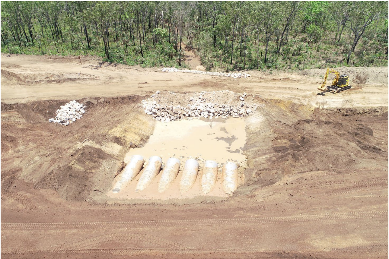
Figure 8: Improved ESC: Improved bunding on the outer edge of the temporary access track to ensure surface water flows don't overtop. Sediment in front of culverts has been dredged out. Additional white rock with clean sand has been installed in front of the temporary crossing to slow water and enable it to filter through the geofab and sand before flowing downstream.
