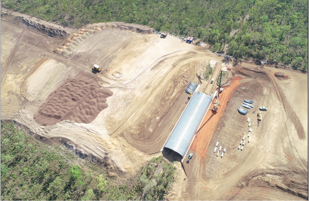
Figure 4A: Sediment controls in place at the Emerald River main channel prior to the sedimentation events.
