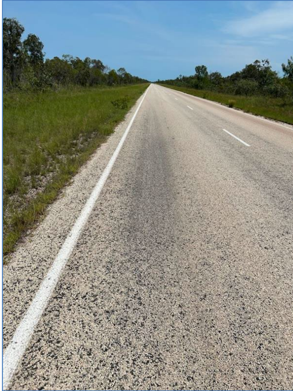
Figure 3: Extent of the second spill heading North towards BBLF (1kg)
