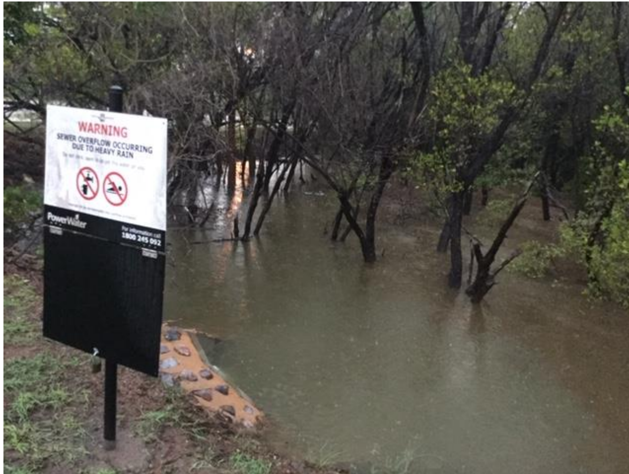
Indicative photo of the sewer overflow relief point on the corner of Rapid Creek Road and Trower Road. Historical photo from 2020.
