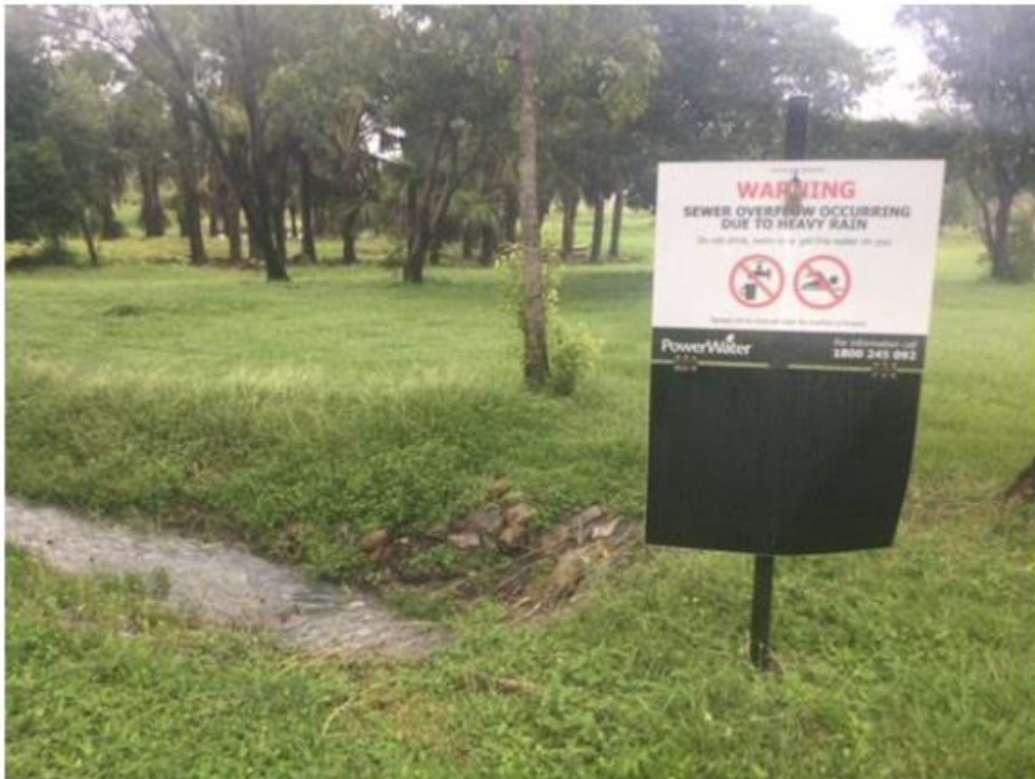
Indicative photo of the sewer overflow relief point at 24 East Point Road. Historical photo from 2021.
