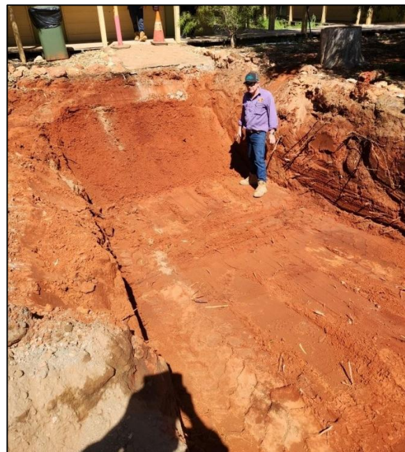
Photograph 2: Deeper excavation area where diesel had pooled
