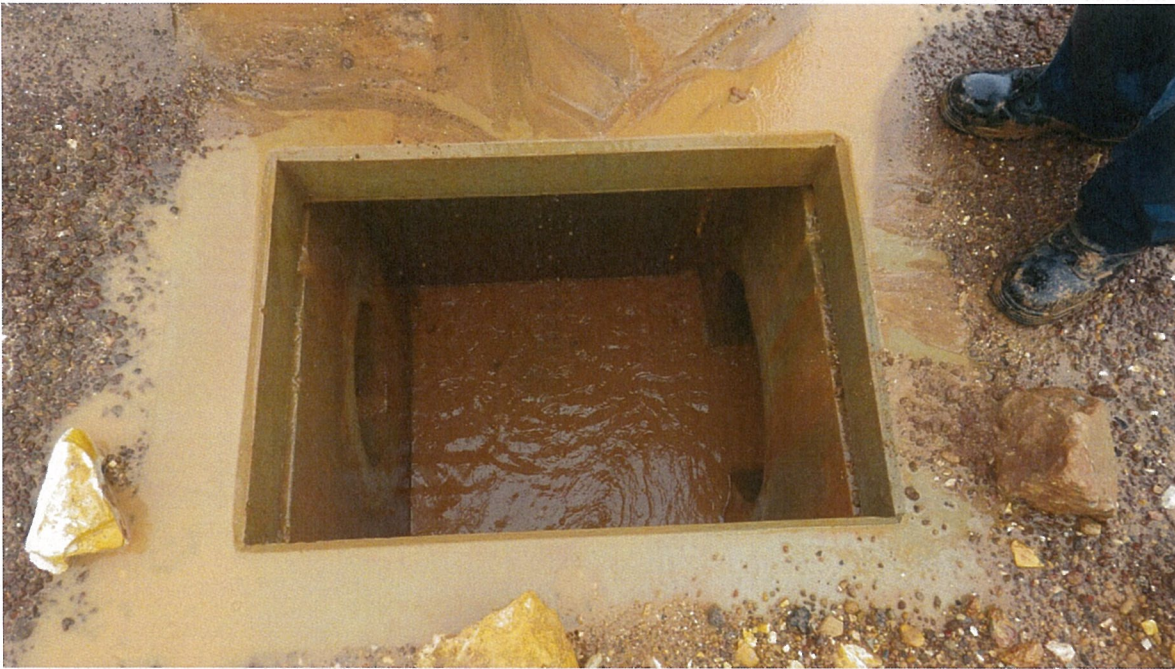
Stormwater entry pit on the premises
