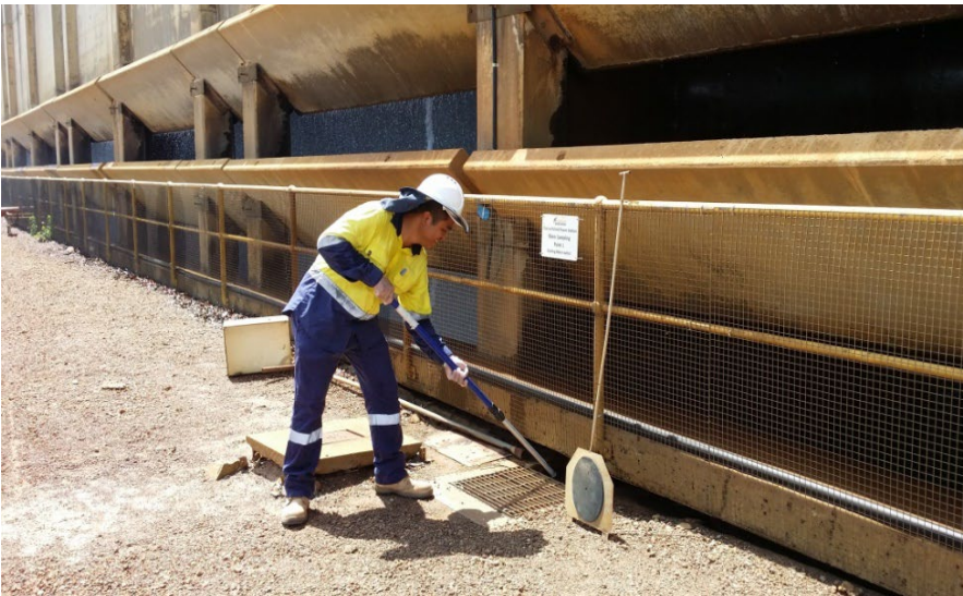
Figure 7: Cooling Tower Discharge Collection Point (ADP1).
