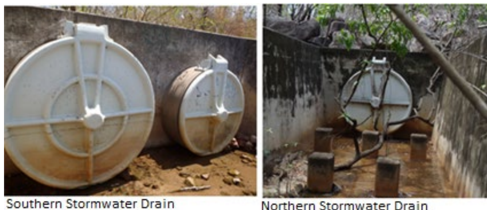
Figure 1: CIPS discharge outlets.
