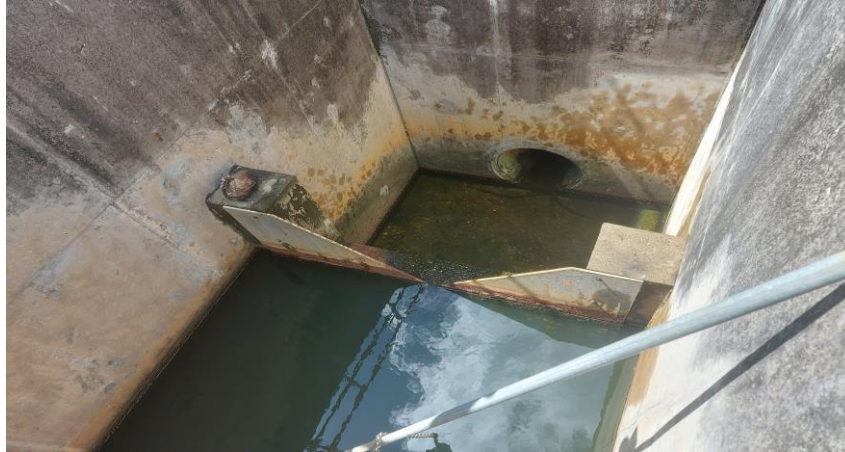
Figure 2: CIPS Authorised Discharge Point 2 (ADP2) or Compliance Point 2.
