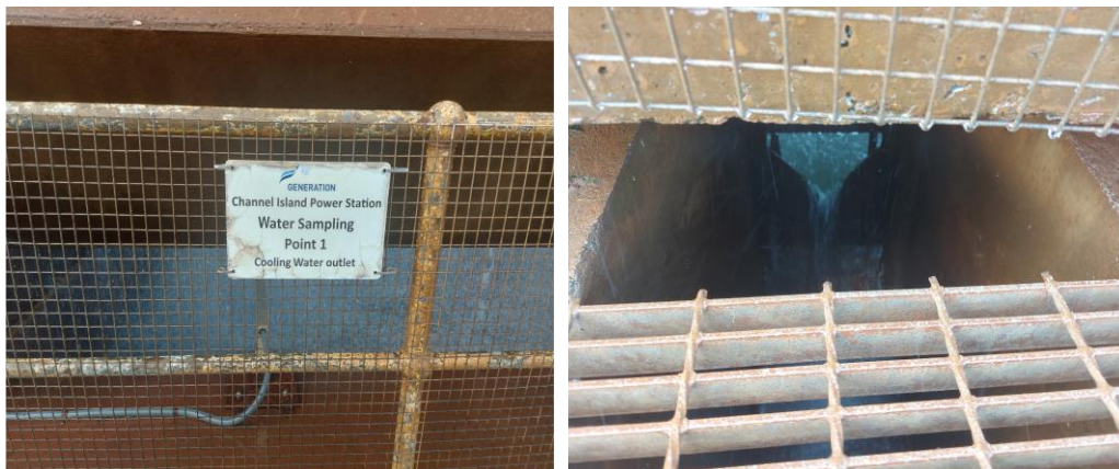
Figure 1: CIPS Authorised Discharge Point 1 (ADP1) or Compliance Point 1.
