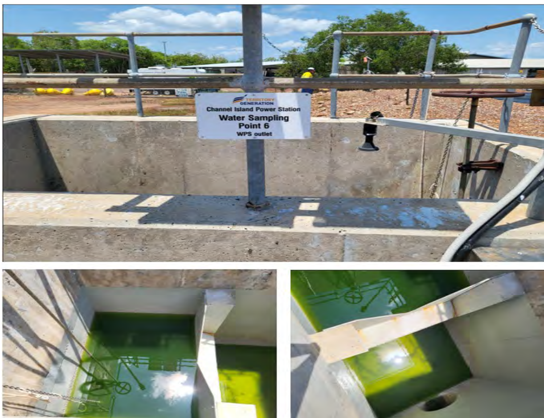
Figure 2: CIPS Authorised Discharge Point 2 (ADP2) or Compliance Point 2.
