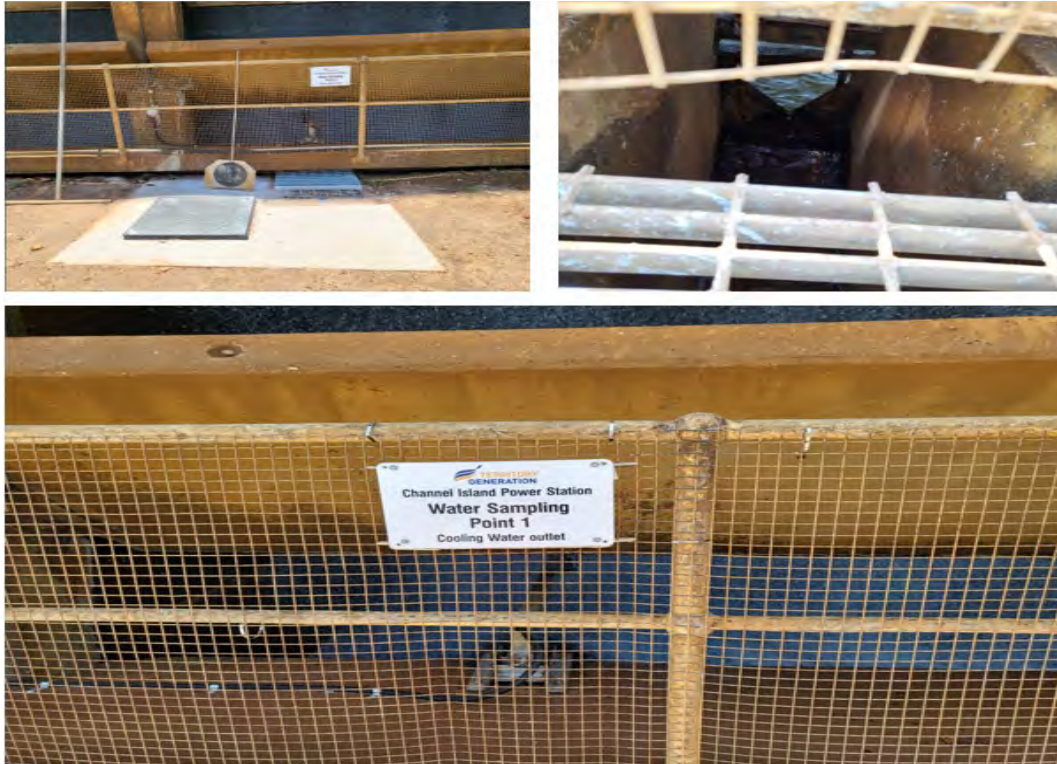
Figure 1: CIPS Authorised Discharge Point 1 (ADP1) or Compliance Point 1.
