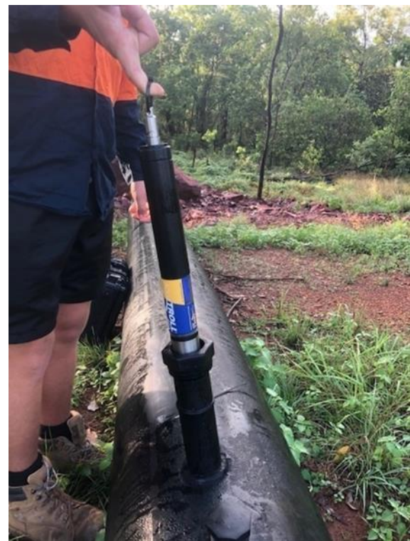
ADP2 (WDL 247 monitoring)-Aqua Troll logger placed in pipe, Rustlers Roost
