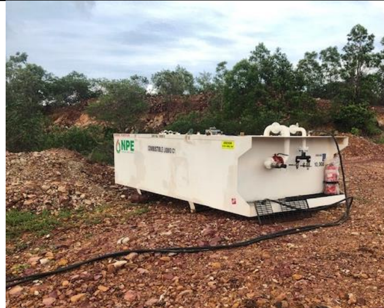
10,000 litre diesel fuel tank and line to generator with leak, Rustlers Roost
