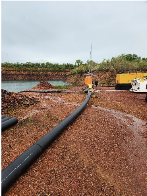
Rustlers Roost Pit Pump infrastructure- electric pumps, 10,000L diesel tank and generator (Jan 2023)
