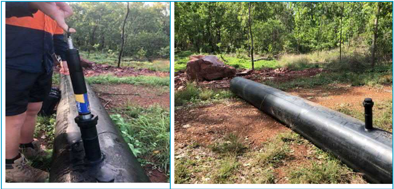
Figure 9 Data logger in discharge pipe (Rustlers Roost WDL 247 Project infrastructure)
