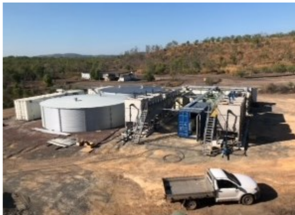
TGPA RO Plant (September 2023)
