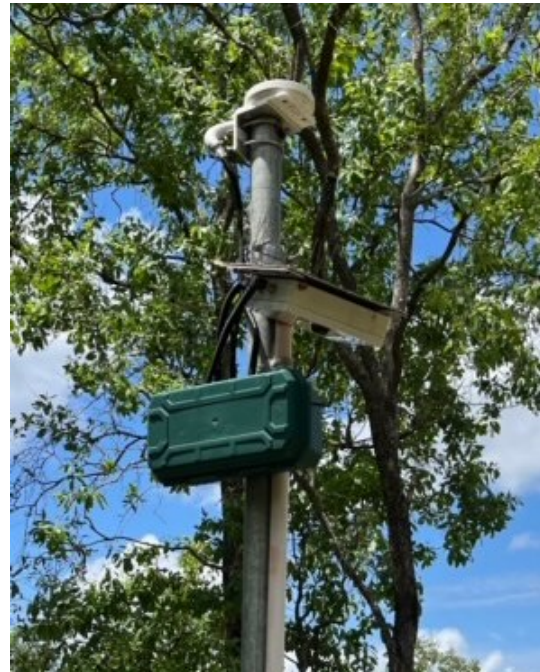
SWTG2 WDL 249 Compliance Point, telemetry station
