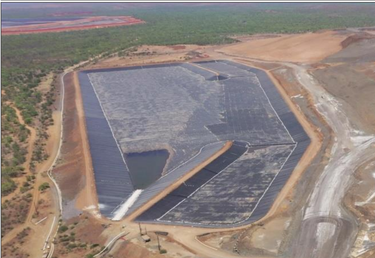
Plate 21: Construction of the TSF Interception Trench (top) and HDPE Lining of SPREAD (bottom)
