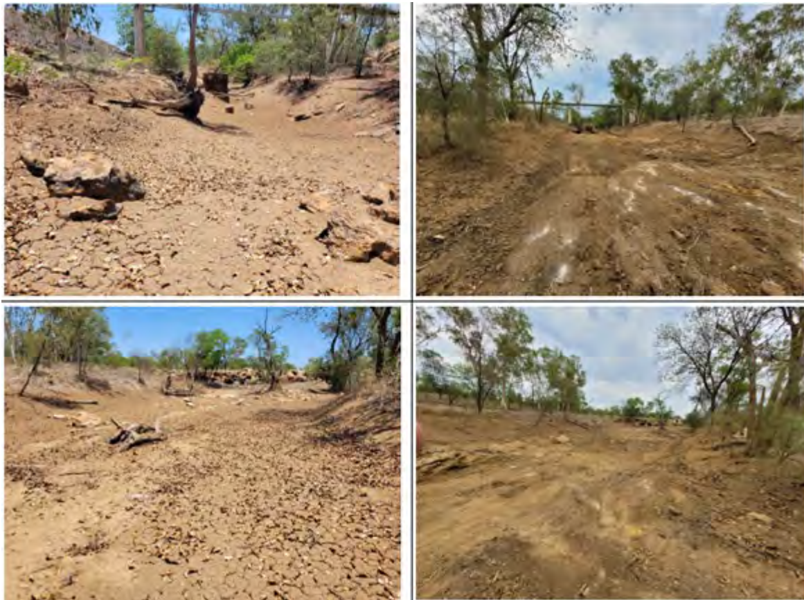
Plate 14: Sediment Removal from Barney Creek and Barney Creek Haul Road Bridge Sump
