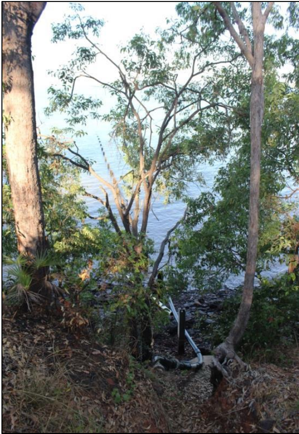
Figure 7. Milikapiti discharge pipeline (PWC 2017)
