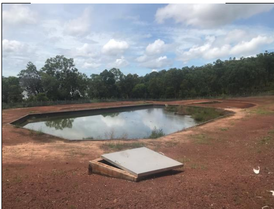
Figure 13: Milikapiti WwTP Wet Season (PWC 2021)
