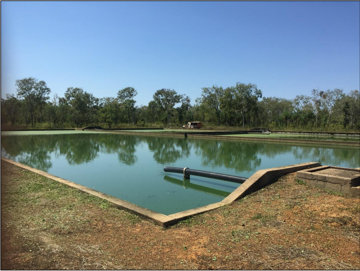
Figure 16: Peppimenarti WwTP (PWC 2021)
