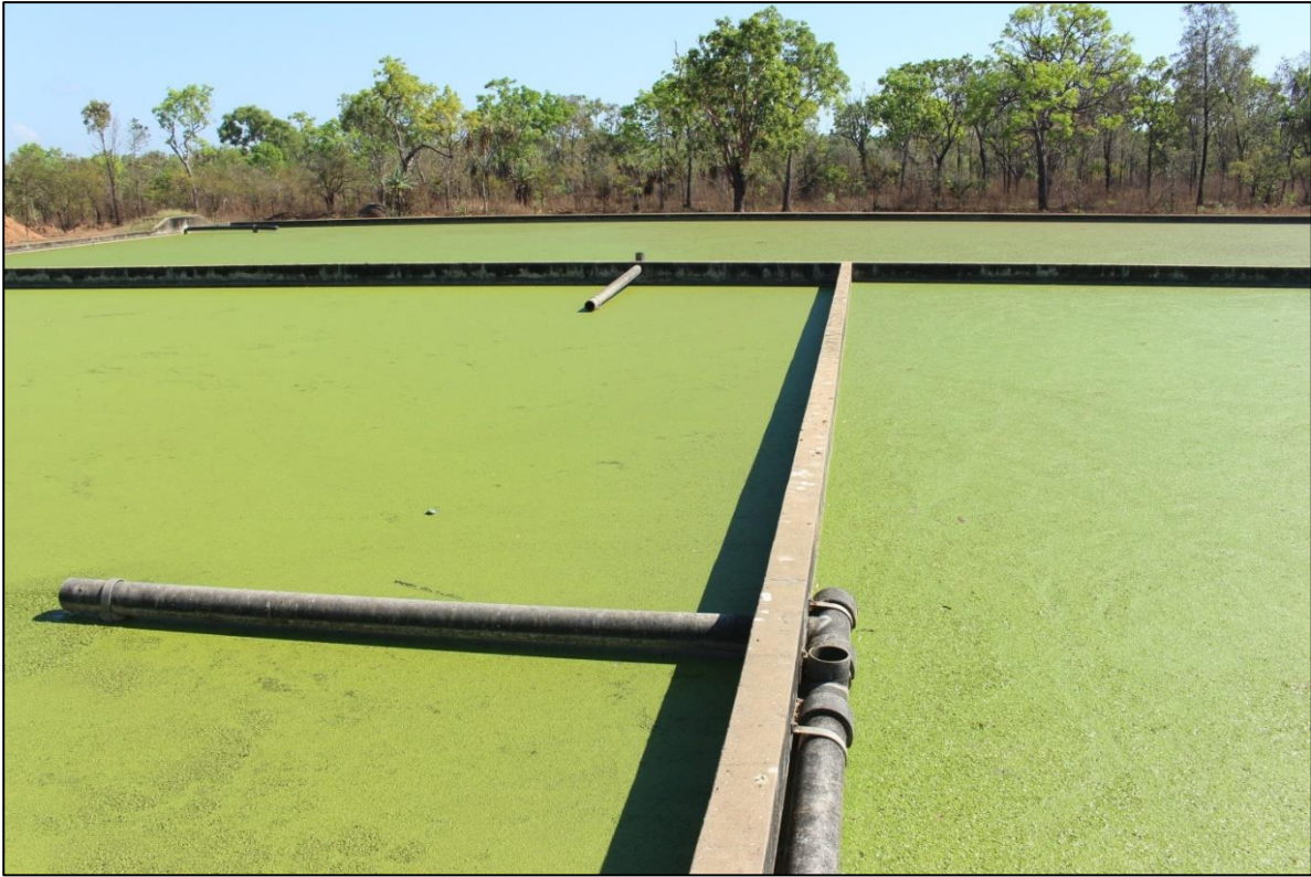
Figure 15: Peppimenarti WwTP (PWC 2017)
