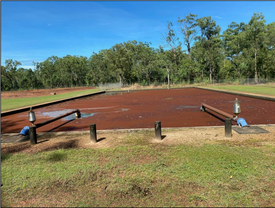
Figure 13. Pirlangimpi WwTP Pond 1 – brown algae observed over time in the pond – Wet Season 2021 (PWC 2021)
