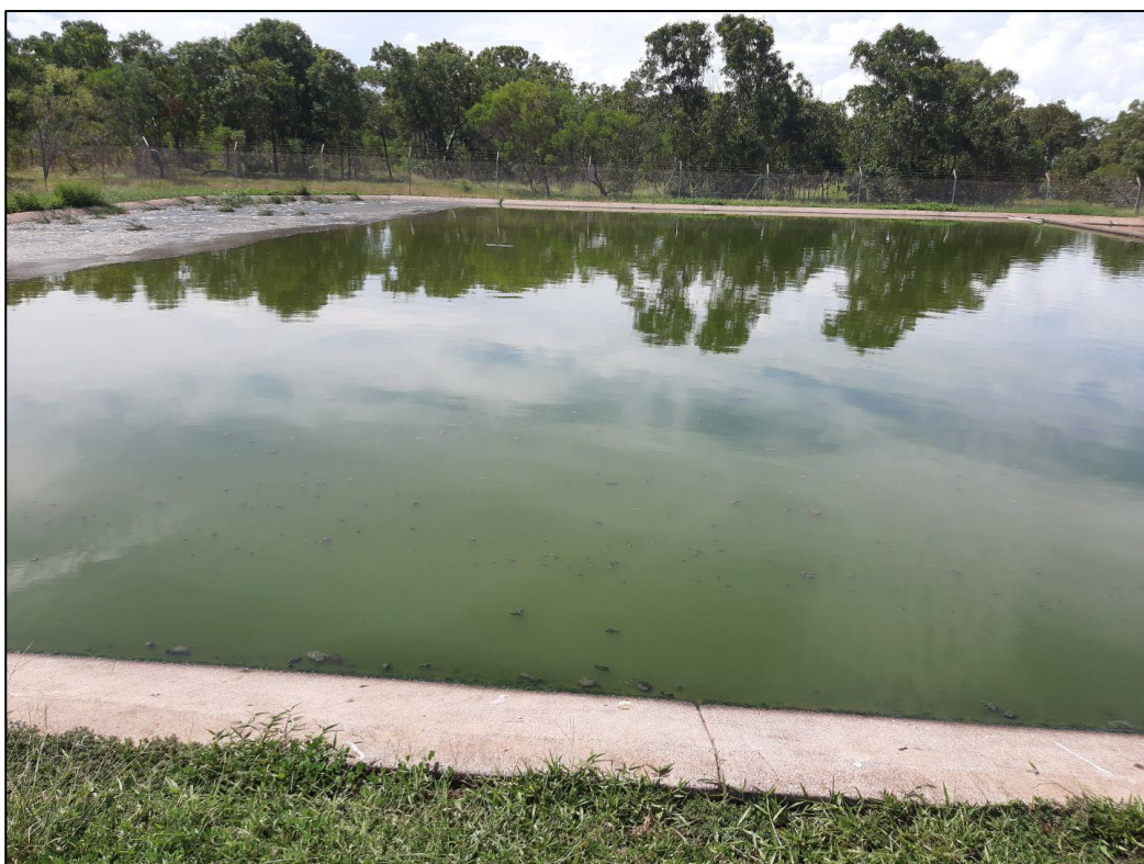
Figure 12. Warruwi WwTP Pond 1 (PWC 2021)
