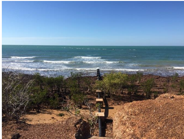
Figure 6. Warruwi WwTP ocean outfall at high tide (PWC 2016)
