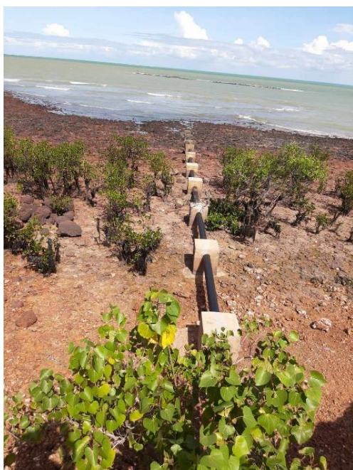
Figure 7. Warruwi WwTP ocean outfall (PWC 2021)
