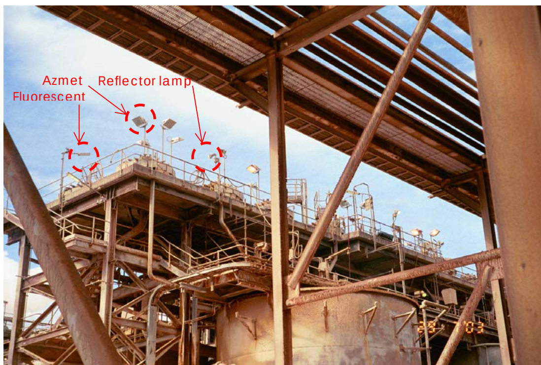
Photo 45. Azmet floodlights, fluorescent and reflector lamps on top of hydrate area.
