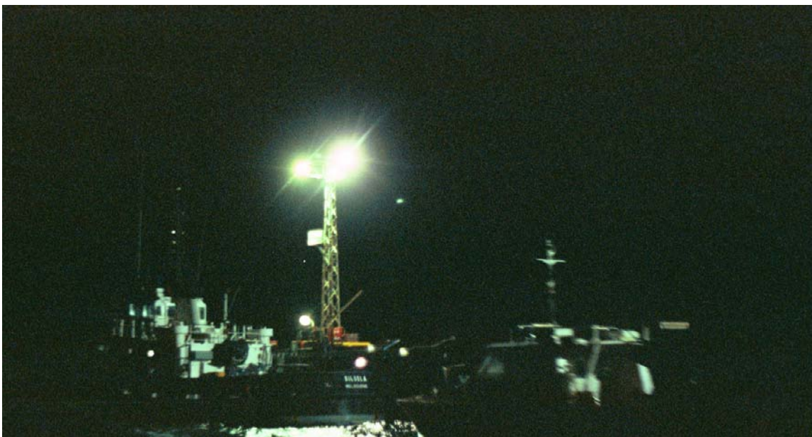
Photo 18. General cargo wharf metal halide floodlighting
