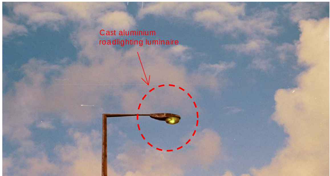
Photo 6. Another type of roadlighting luminaire – mercury vapour.
