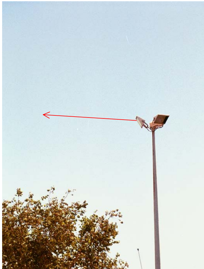
Photo 7. Main car park – EYE Azmet floodlights. One floodlight aimed with the peak at or above horizontal.
