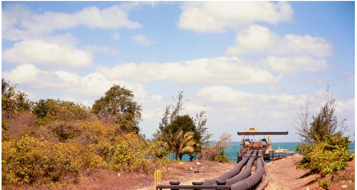
Photo 10. Pumping station adjacent Galupa settlement.
