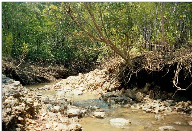
Creek bank erosion from release of pond water into natural mangrove areas
