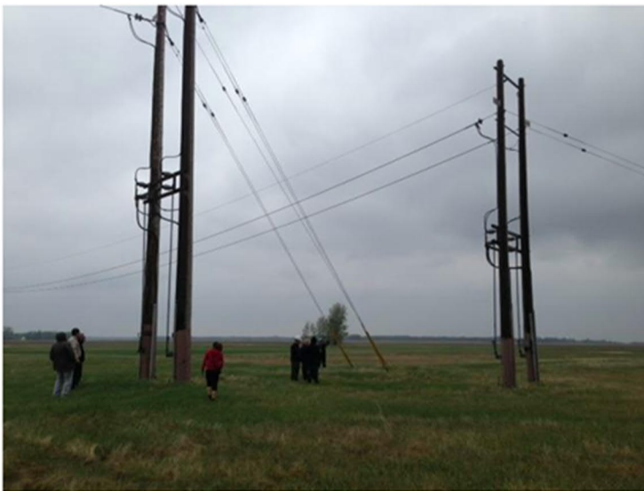
Figure 2-30. An Electrode Site Without a fence and electrode switches mounted on poles [CIGRE TB 675 Figure 7.4]
