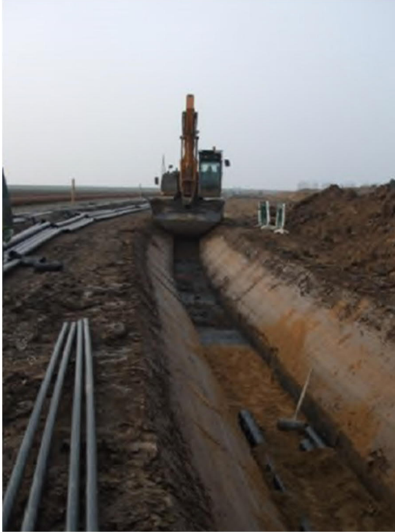
Figure 2-36 – Photo of sub soil excavation in a trench with side slopes (Source: Prysmian)
