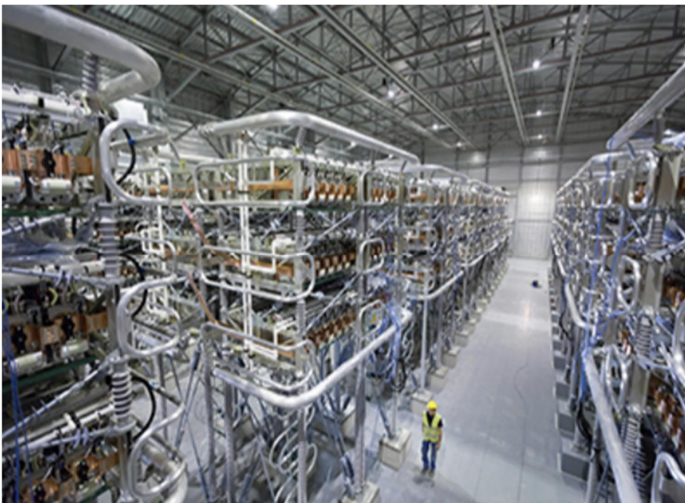
Figure 2-31. Internal view of a Voltage Source Converter (Source ABB Power Grids Pty Limited)
