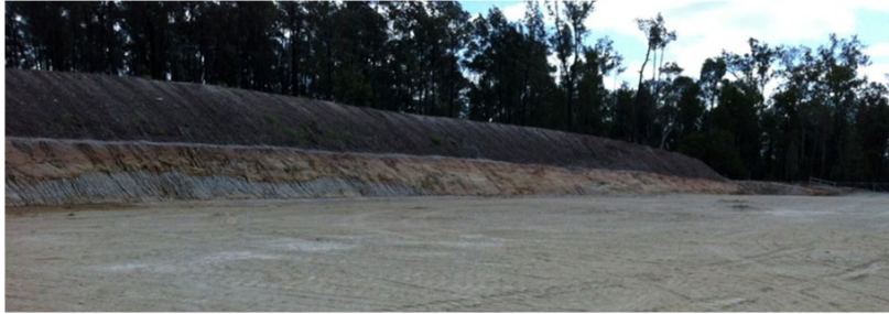
Figure 8: Topsoil Windrow Above the Cut Batter used to Divert Clean Water away from the Well Pad
