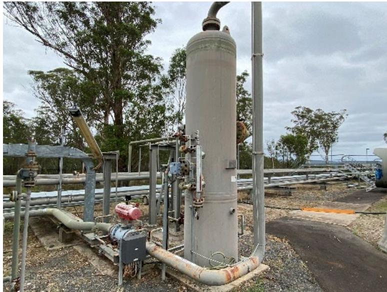
Figure 33: Indicative discharge scrubber
