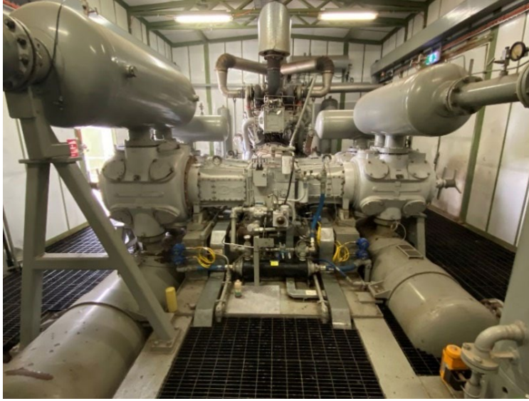
Figure 31: Indicative compressor unit
