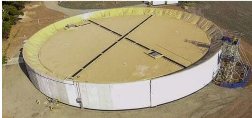
Figure 36: Indicative Water/wastewater tank, fitted with cover
