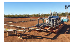
Image: Separator on Carpentaria site
