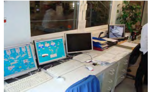
Plate 3-8 Control room of typical hydraulic backfill plant
