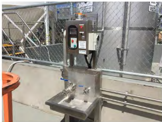
03 Chemical Transfer hose connection and tanker operators local control panel
