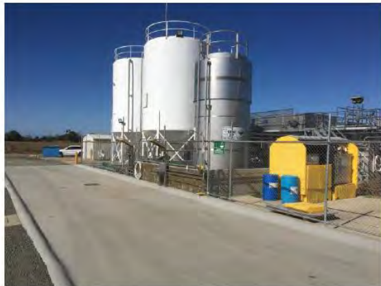
01 Chemical Tanker delivery bay
