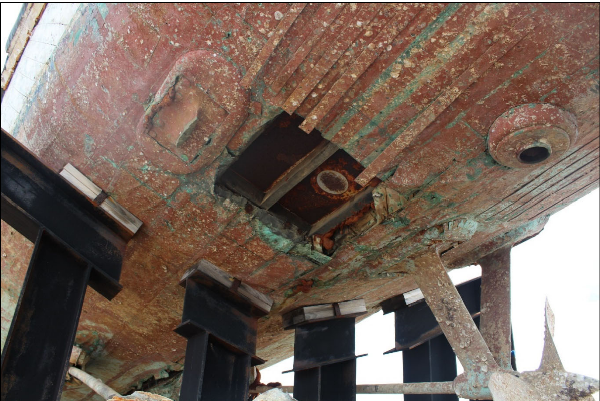
Figure 19: Image of HDML 1321 on hardstand. Note damage below the waterline and separation of rudder from the rudder shaft
