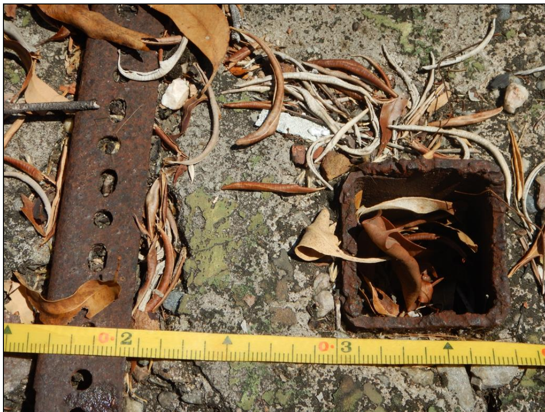
Figure 20. Site 2 – Slab 4. Central post-hole and wall footing, close up. Scale in 1cms.
