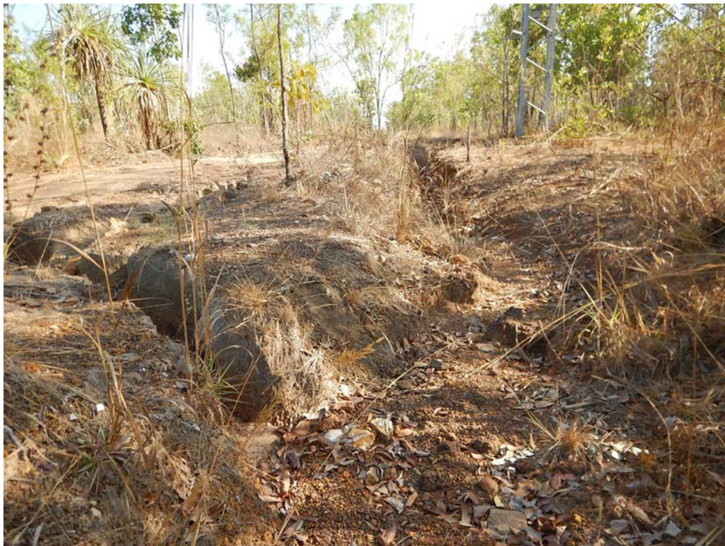
Figure 2-6. Image showing gully erosion next to dirt road
