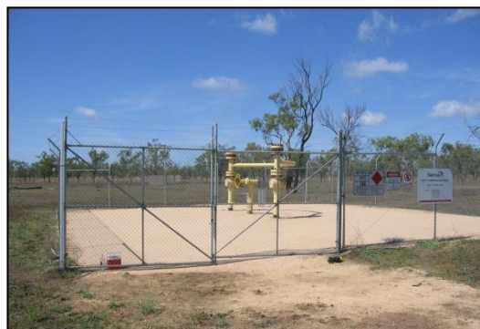
A mainline valve. W. Mathieson
