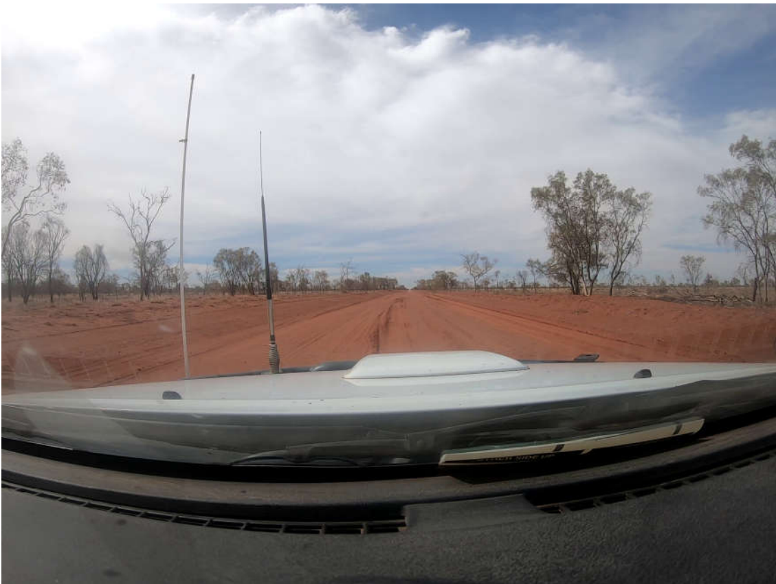
Photo 17 – Poor pavement with low profile and no stormwater egress
