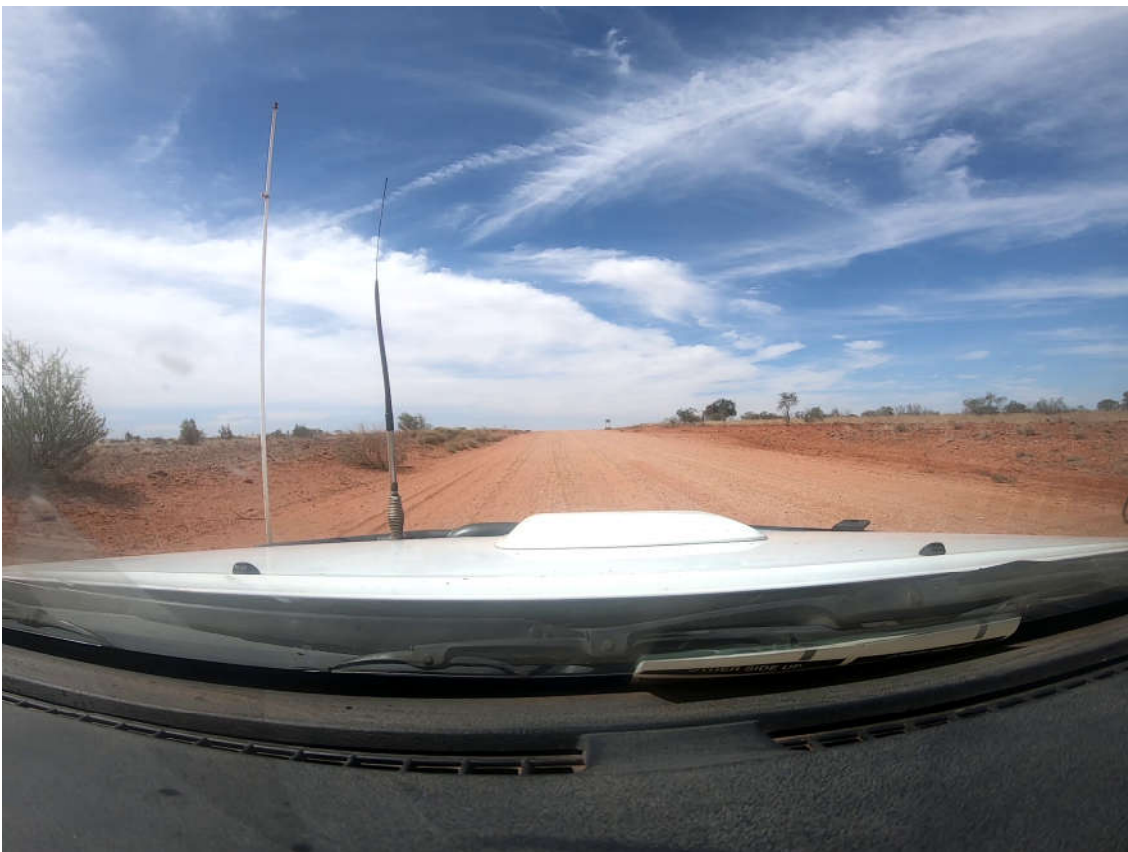
Photo 11 – Poor sight distance to crest at Ch. 273.20km
