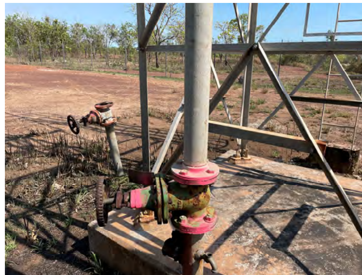
Photo 22 Water tank slab, north of RA shed, ACM pipe gaskets marked in pink
