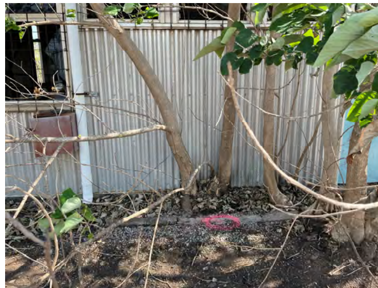
Photo 14 Southern external wall, ACM fragment marked in pink
