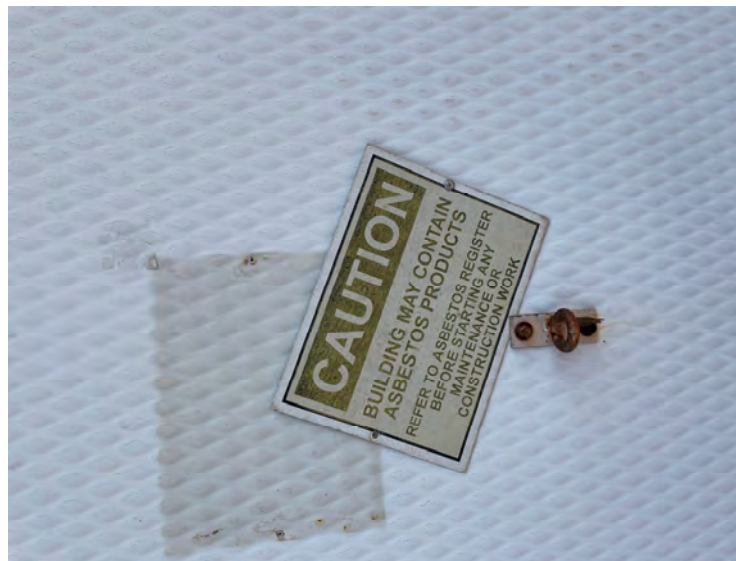
Photo 12 Existing SMALL BUILDING, asbestos caution
