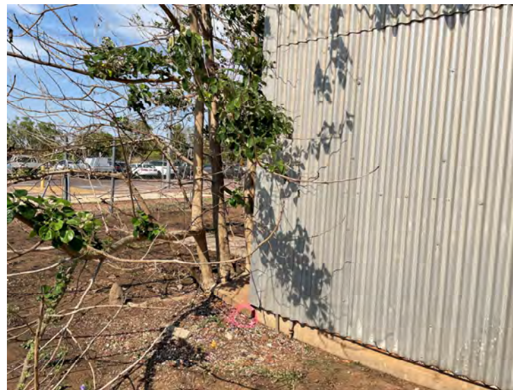
Photo 16 South eastern corner, external wall, ACM fragment marked in pink
