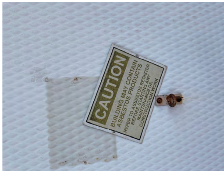
Photo 12 Existing SMALL BUILDING, asbestos caution
