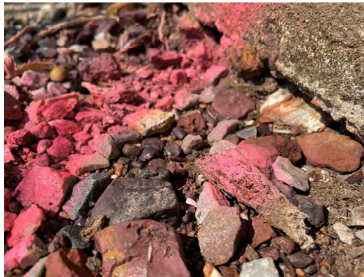
Photo 18 South eastern corner, external wall, ACM fragment marked in pink
