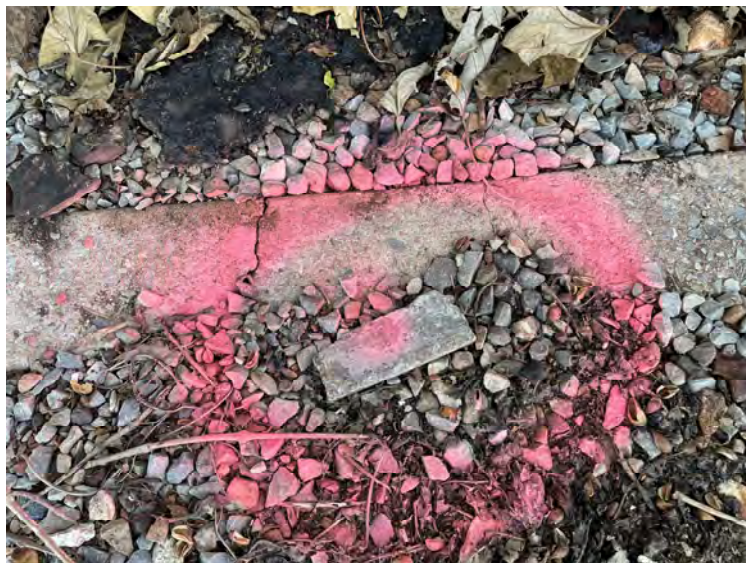
Photo 15 Southern external wall, ACM fragment marked in pink Sample M-AS1
