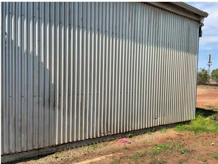
Photo 19 Northern perimeter, external wall, ACM fragment marked in pink
