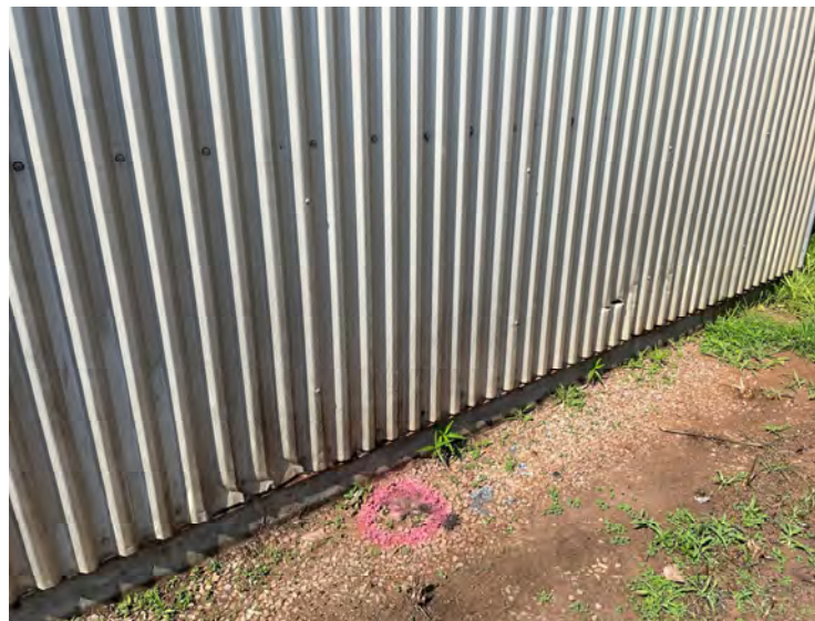
Photo 20 Northern perimeter, external wall, ACM fragment marked in pink
