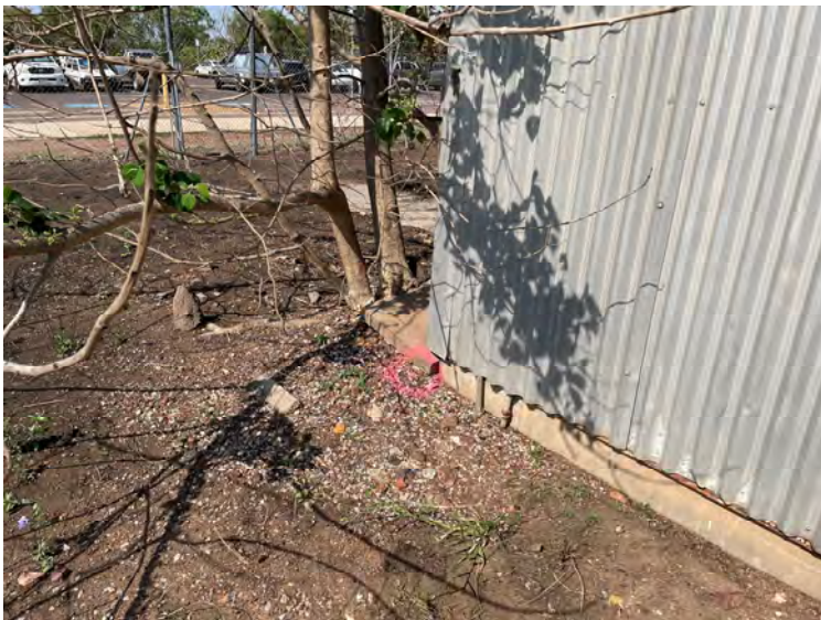
Photo 17 South eastern corner, external wall, ACM fragment marked in pink
