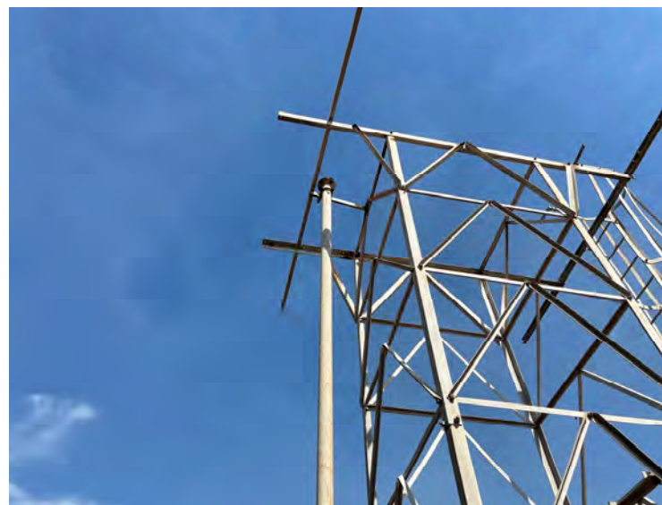
Photo 24 Water tank tower, north of RA shed, assumed ACM pipe gaskets
