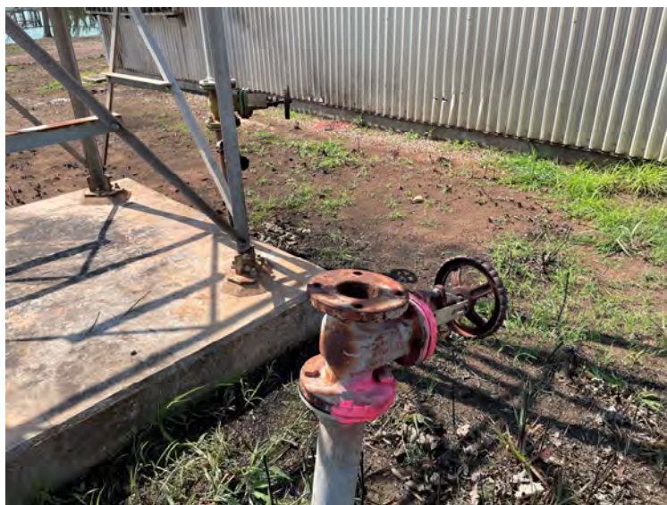
Photo 23 Water tank slab, north of RA shed, ACM pipe gaskets marked in pink
