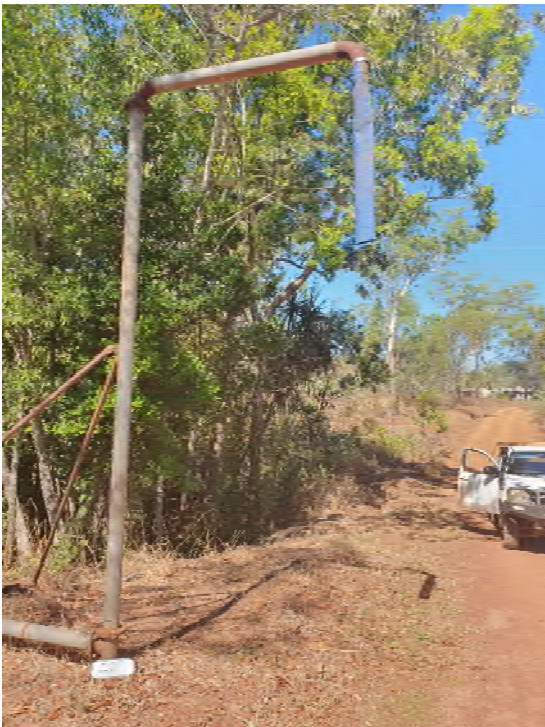
Taracumbi Creek at outstation Standpipe
