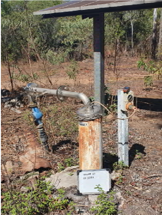
Taracumbi Outstation Bore RN32883
