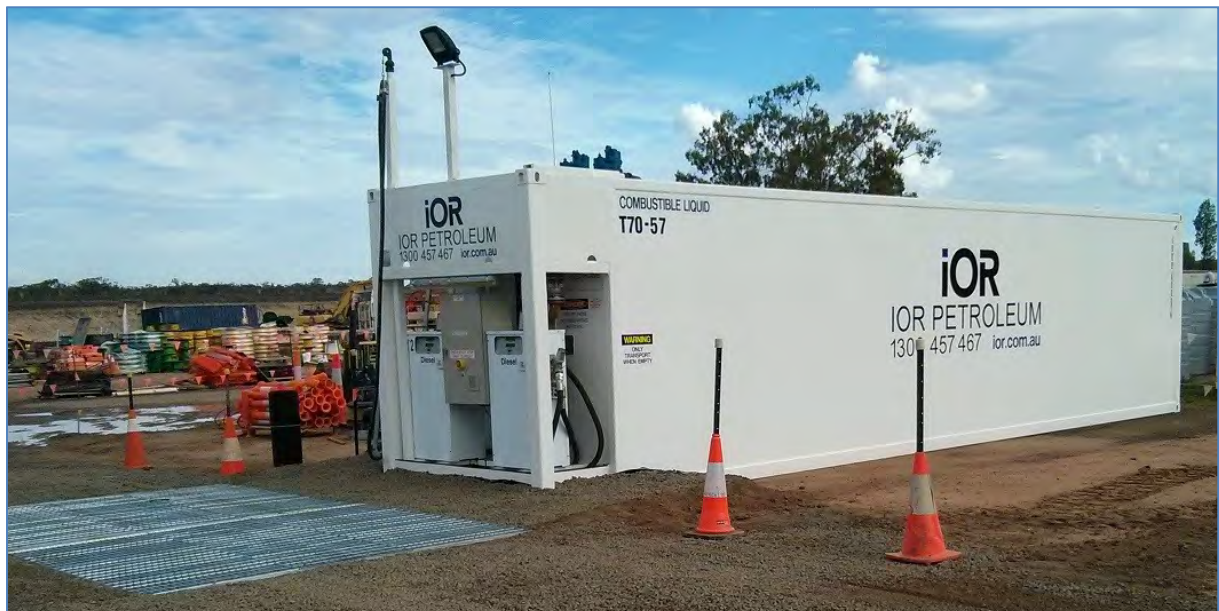
Plate 2-2 Example of 85,000 L self-bunded tank
