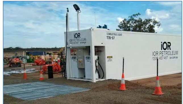
Plate 13-1 Example of 85,000 L self-bunded tank
