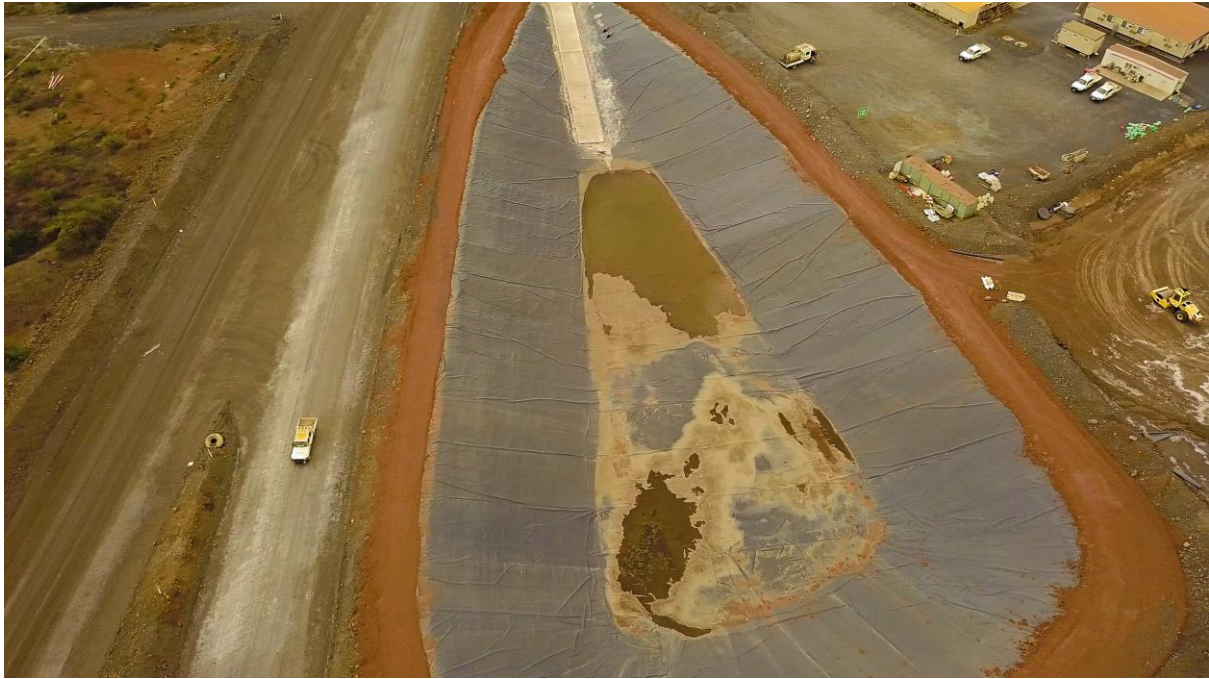
Figure 3-5 New HDPE-lined MIA Sump
