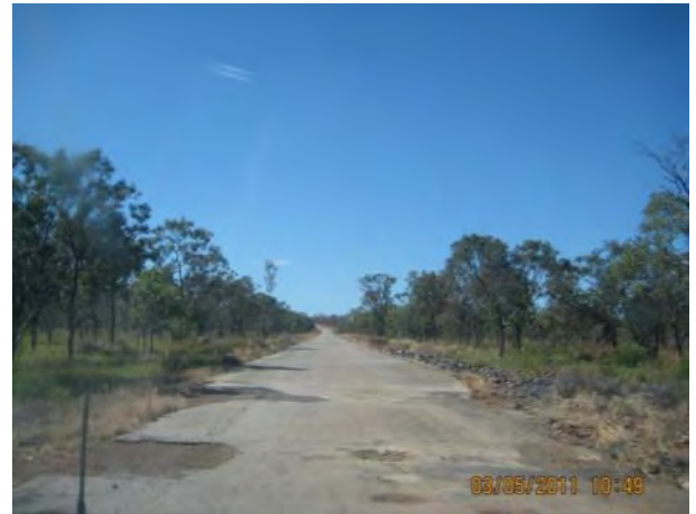
Figure 8 Jatbula Road (Mine Access Road) cross section – localised poor pavement condition, view to north
