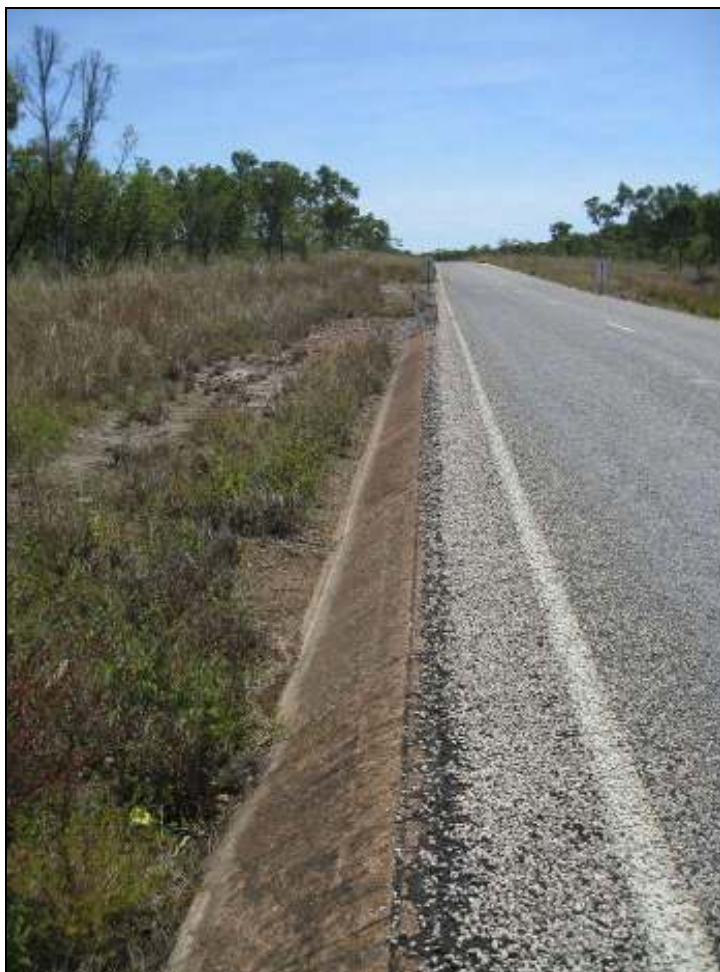
Figure 6 Narrow carriageway with sudden drop-off at causeway
