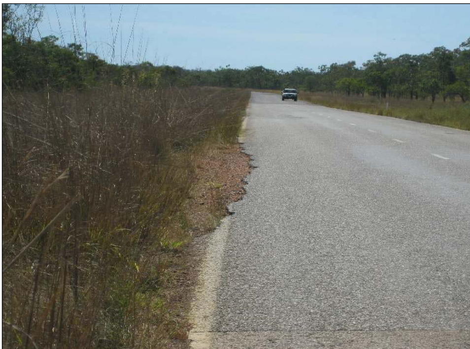
Figure 8-3 Example of uneven surface and incorrect camber
