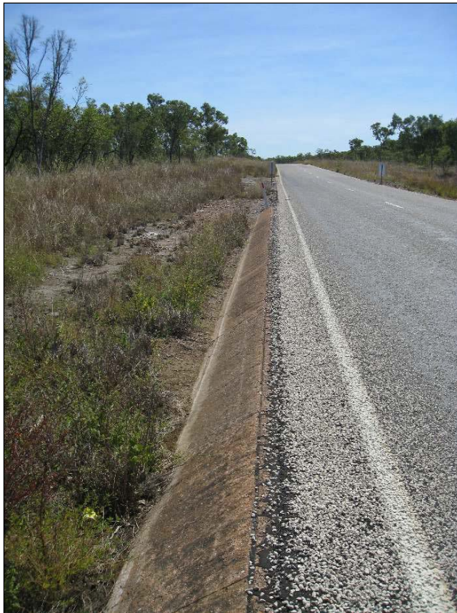
Figure 8-4 Narrow carriageway with sudden drop-off at causeway
