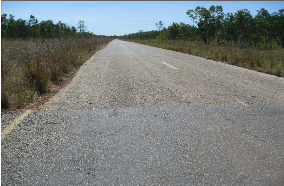
Figure 8-2 Example of uneven surface and incorrect camber
