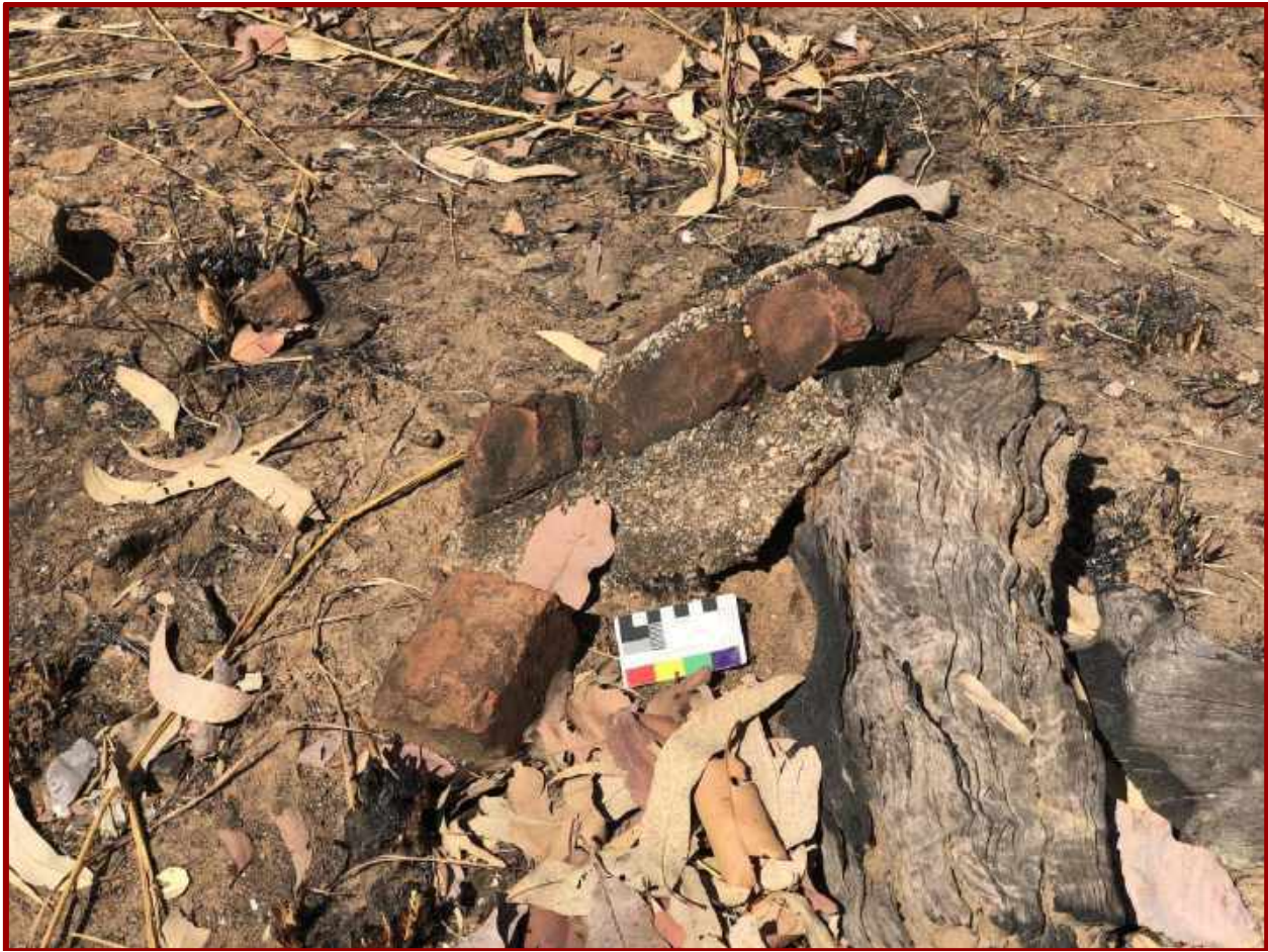
Figure 97: Remains of disturbed bricks and mortar
