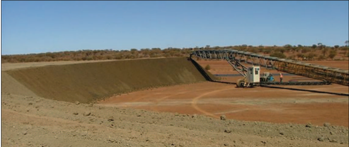
Plate 4.5 – A Typical Radial Stacker on Heap Leach Pad
